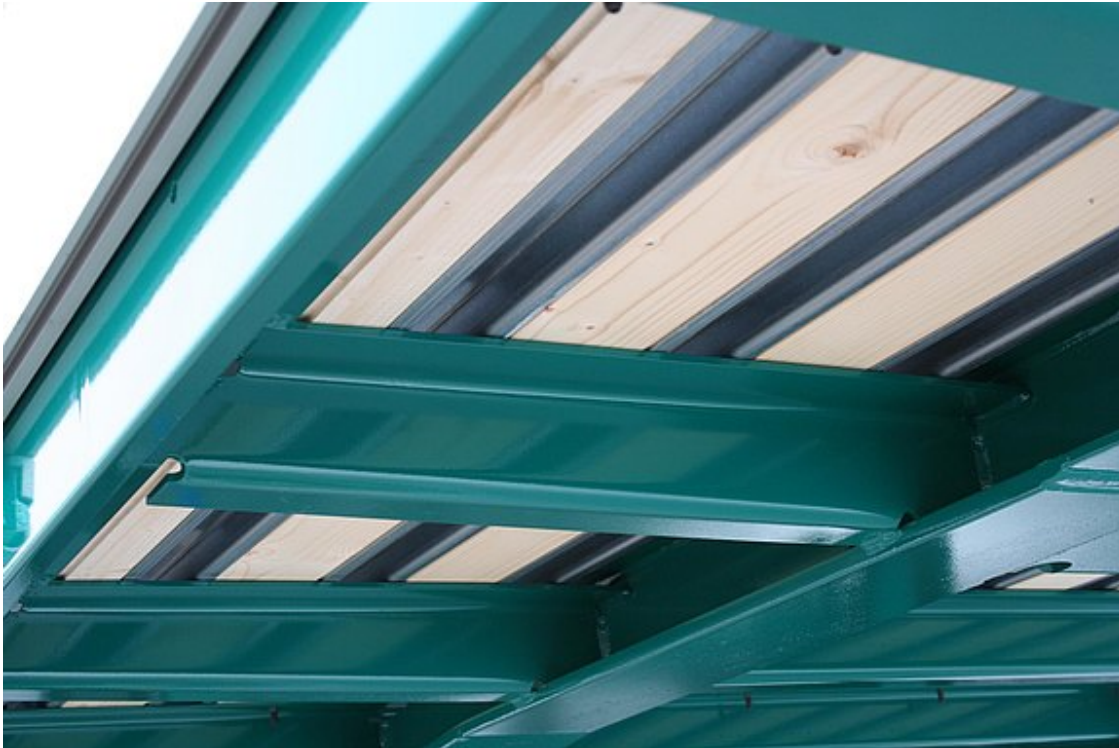
Double floor consisting of subfloor with integrated steel omega profiles beneath resin-coated wear floor (stacker axle load: 7 t)
