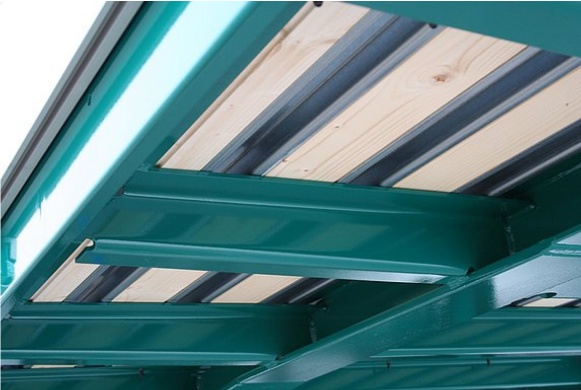
Double floor consisting of subfloor with integrated steel omega profiles beneath resin-coated wear floor (stacker axle load: 5,460 kg)
