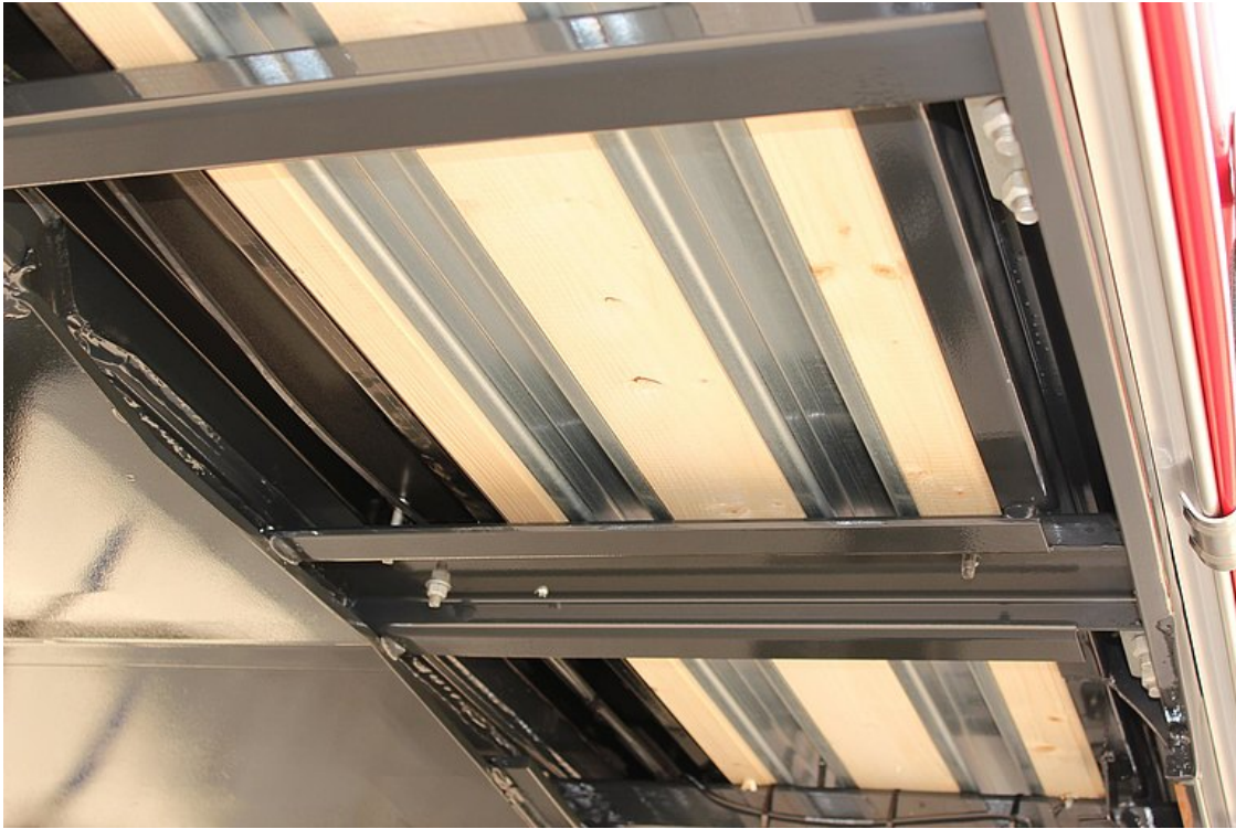
Double floor consisting of subfloor with integrated aluminium omega profiles beneath resin-coated wear floor (stacker axle load: 7 t)
