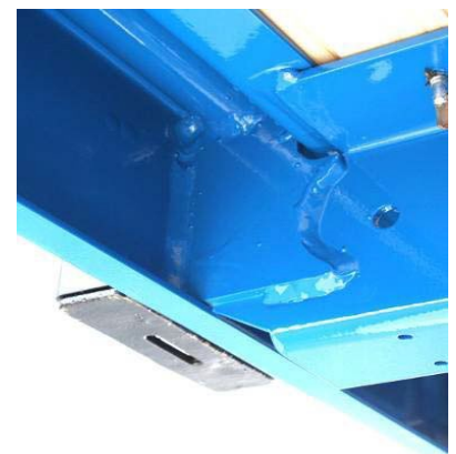
Interior stanchion bearings: Check the weld seams for cracks
