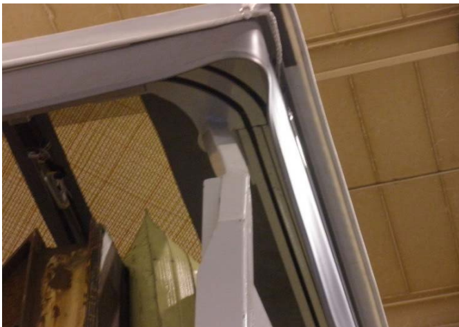
Edscha Eco variant with fixed rear wall: Check rear corner post link and bend for damages, cracked weld seams etc.
