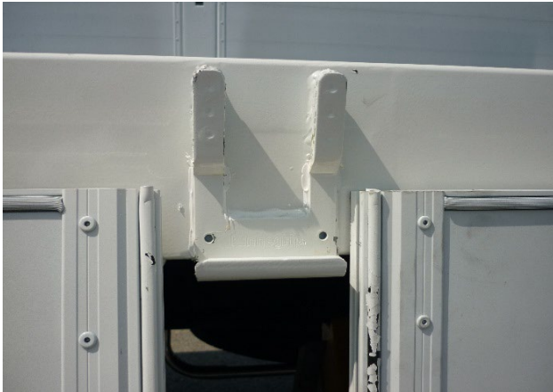
Stanchion bearings: Check the weld seams for cracks
